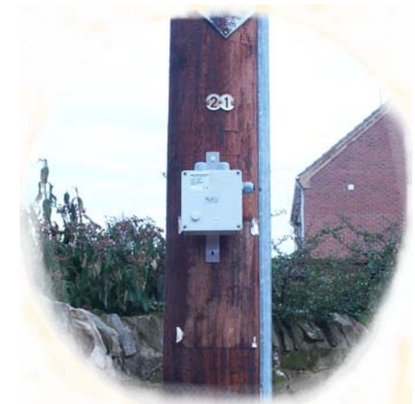
Pole mounted M61
